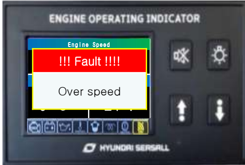
Case 1 Safety Fault list (refer to chart next page) 1. Over speed 2. Water temperature 3. Oil pressure
